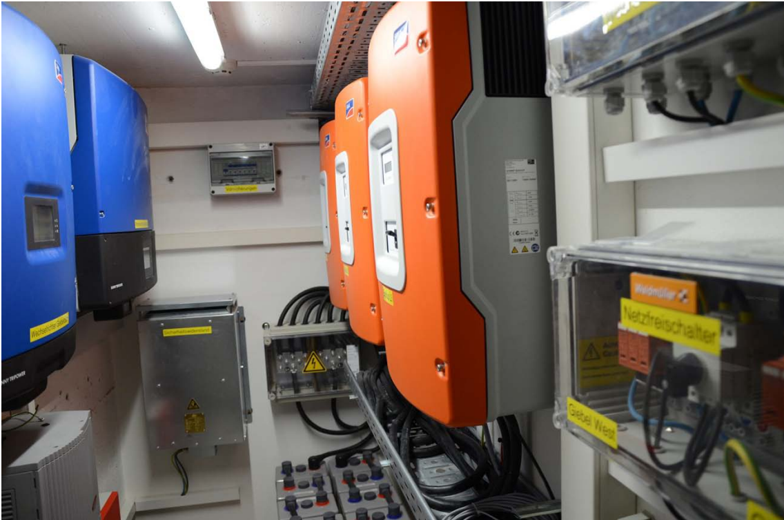
Picture 2: Storage system and converters, source: Elektro Wultschnig
