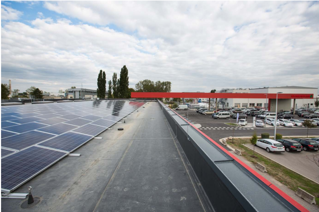
Picture 4: PV panels on the roof; source: SPAR / Johannes Brunnbauer
