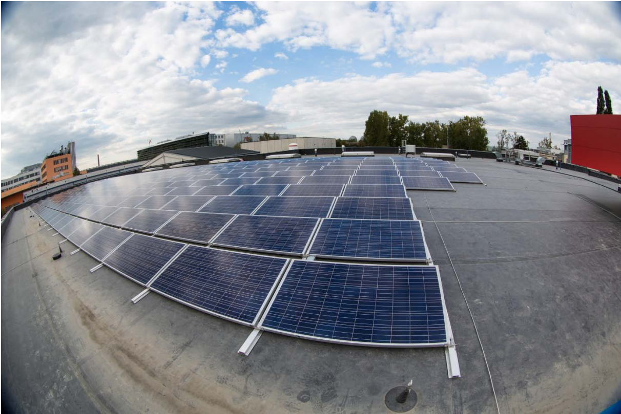
Picture 2: PV panels on the roof; source: SPAR / Johannes Brunnbauer
